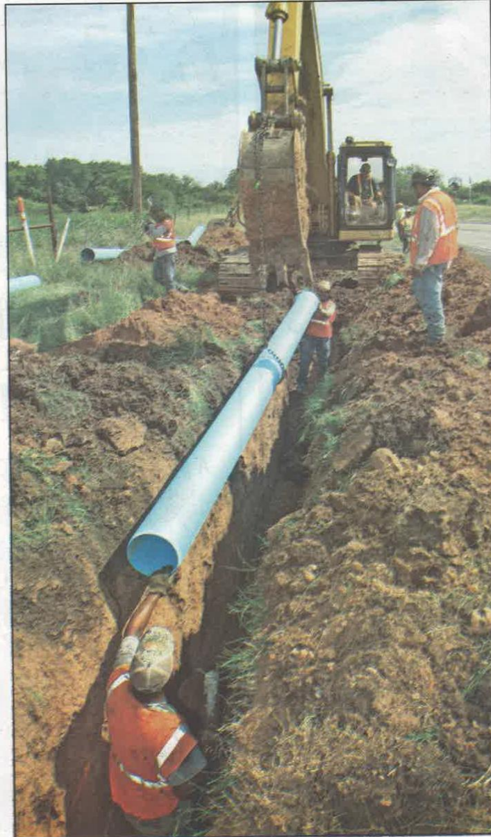
Workers lay the line for the San Saba to Goldthwaite water supply line.
