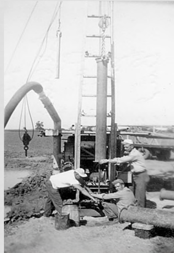
Workers with the Steingard & Schmidt Irrigation Well Co. rig, York County, NE.
