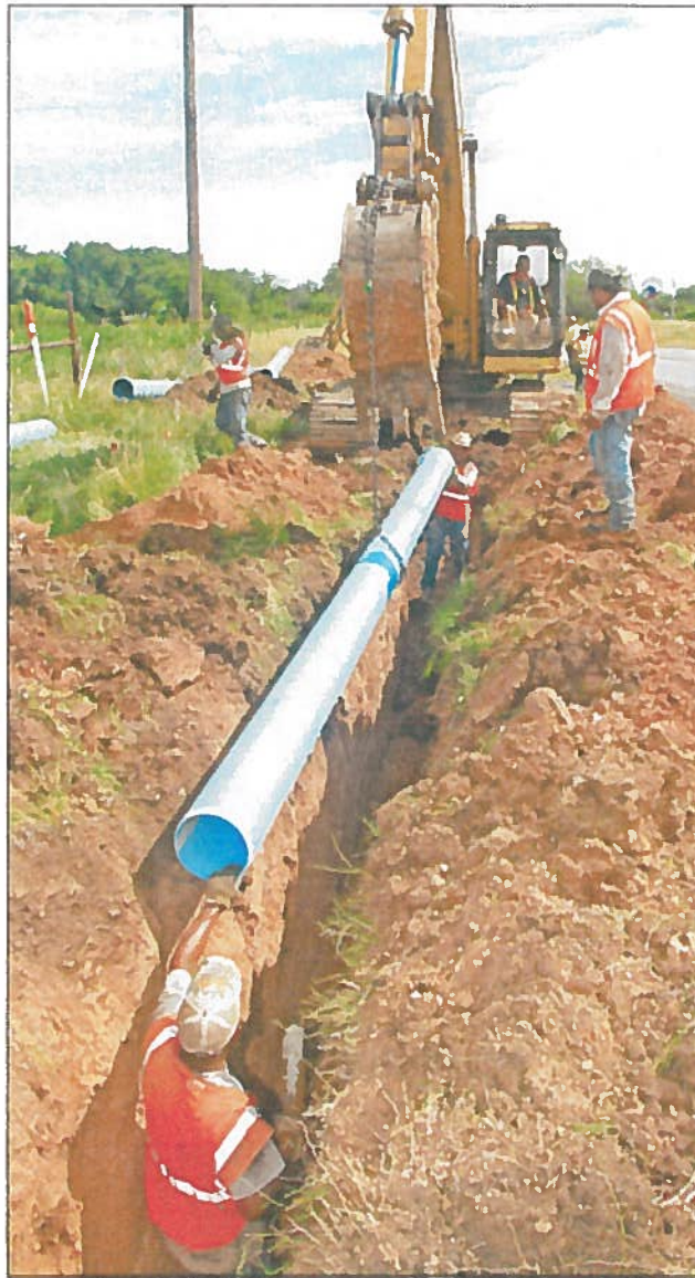
Workers lay the line for the San Saba to Goldthwaite water supply line.
